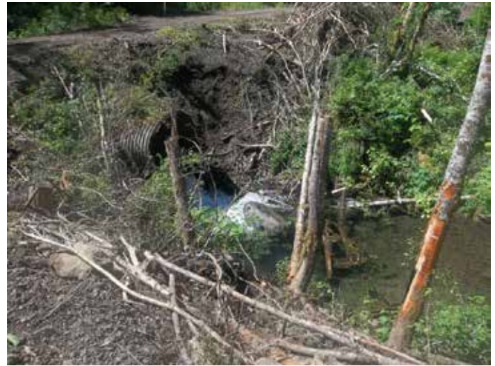
Before: The 10-foot diameter culvert threatened to fail and let loose 2000 cubic yards of sediment into the creek - enough to fill over 150 large dump trucks. Photo: Carl Chastain
